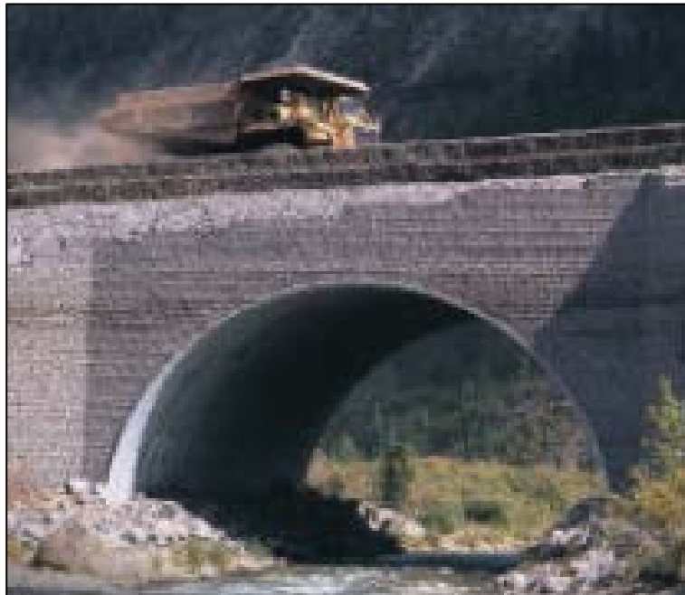
Figure 14-7: Example arch culvert stream crossing photo (Source: www.ail.ca)
